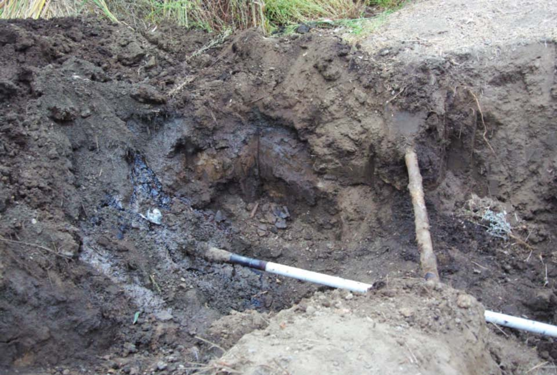
The leak occurred in a single 2" diameter pipe that had recently been tested for leaks.
